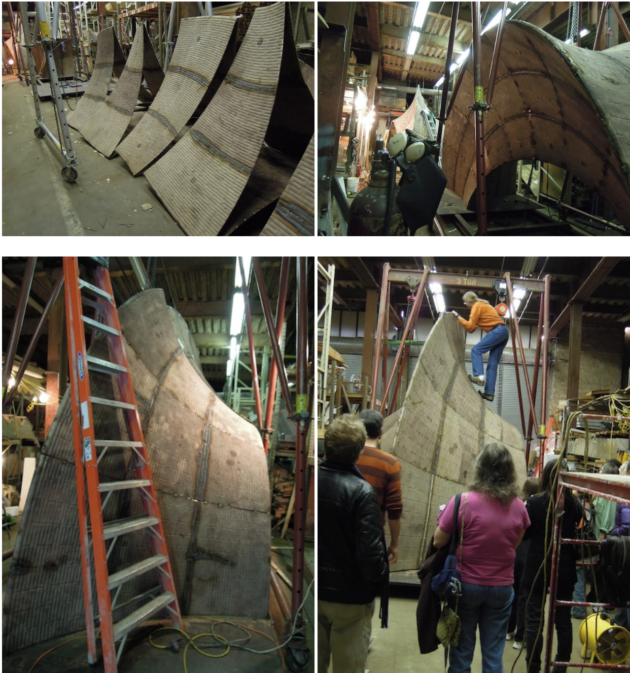
The top and bottom halves will be assembled outside the Torus Assembly Building in Baltimore before dis-assembly and shipping the two halves for re-assembly in Stony Brook •••
